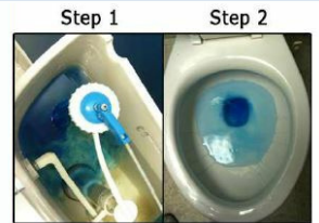
Step 1: Add 1 tablet to the tank. Let sit for 10 minutes. Step 2: If the bowl turns blue or blue streaks appear, a leak is discovered.
